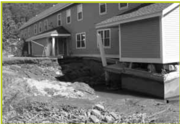
Flooding undermines the foundation in this 4-unit condo in Proctorsville
