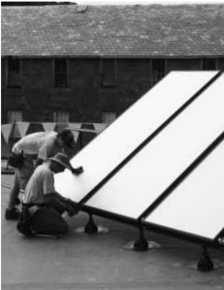
Saving energy and money; SolarWrights' crew install domestic hot water solar panels atop the Daly Shoe Building in Brattleboro.
